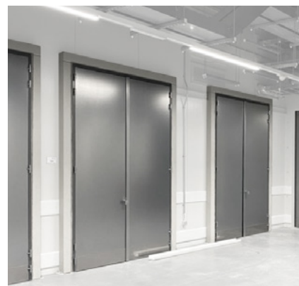
Datacenter / Local IT
